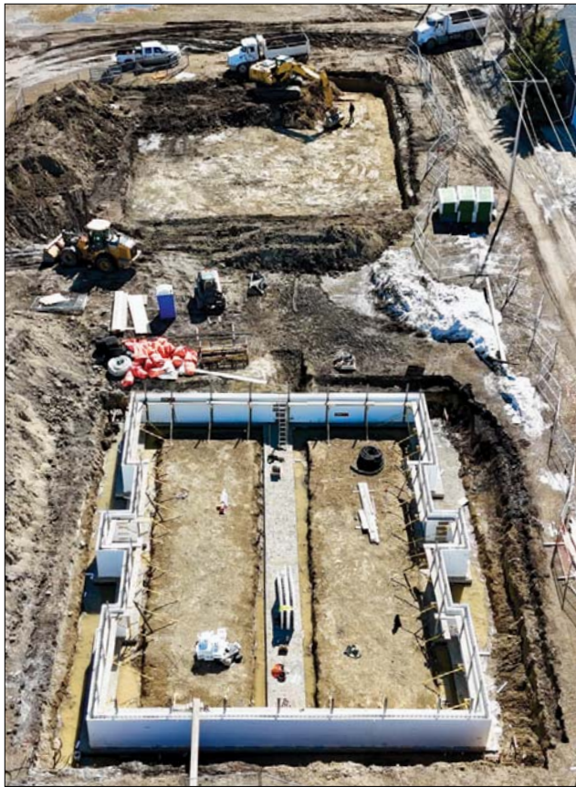
Keller Developments was working on construction of two apartment buildings in Moosomin. In this photo, work is being done on the foundation of one of the buildings, as work got underway on excavating the foundation for the second building.
