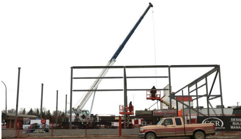
The steel started to go up on Borderland Co-op's new food store in Moosomin last week. The 30,000 square foot store is being built at the corner of Birtle Street and Broadway Avenue and is slated to be completed in early 2025.
