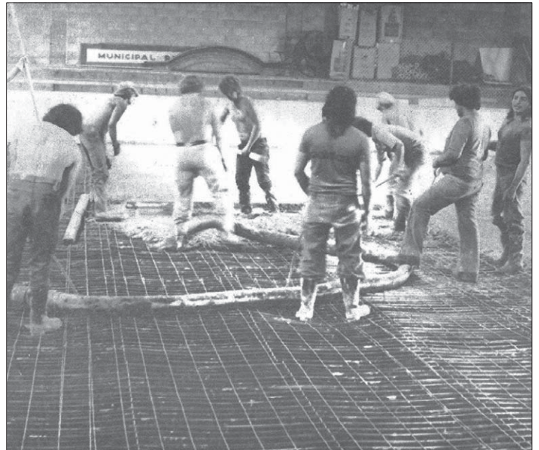
Seen here are members of Western Concrete Finishers Ltd. finishing the concrete floor in the Moosomin Communiplex. This photo appeared in the World-Spectator 30 years ago in 1980.
