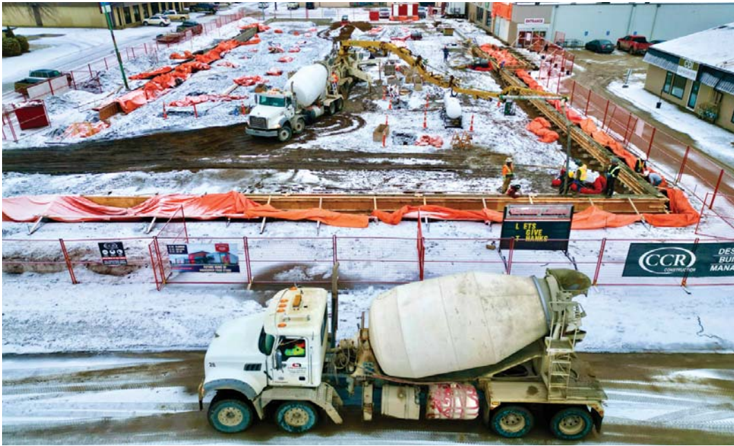
Construction continues on the new Borderland Co-op Food Store being built in Moosomin. This aerial shot taken by Kevin Weedmark shows some of the construction work with the current grocery store in back. Once the new store is built, the current store will be demolished and that area will be used for parking.
