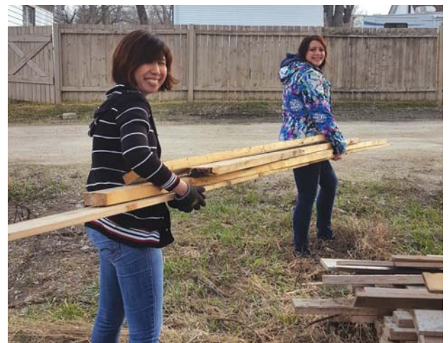
Karen Bargentinos and Andie Hodgson hauling lumber and doing building clean up the McNaughton Building restoration project.
