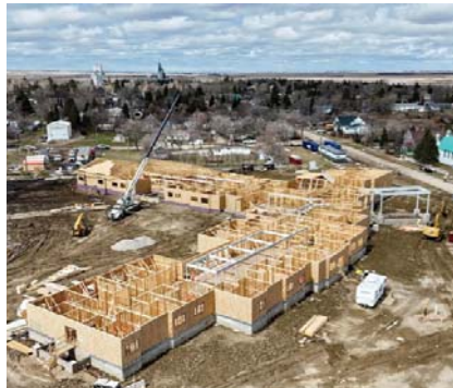
The new 33-bed long term care facility taking shape at Grenfell. The facility is 25% complete.
