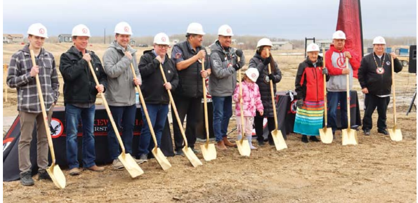
Above, members from Kahkewistahaw First Nation, Corex Construction, BCL Engineering, SAL Engineering and Indigenous Services Canada at the Sod turning on the site of the new water treatment plant.
