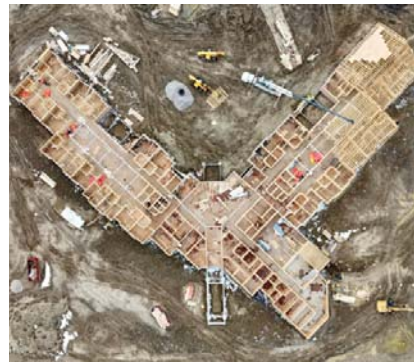
The new 33-bed long-term care facility under construction in Grenfell. We have reduced the community cost of new facilities like this to 10% down from 20% under the NDP. It was a ridiculously high 35%.
